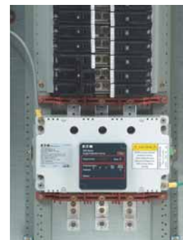
In this installation, the SPD Series is mounted directly to the panelboard's bus bars. This type of installation will provide the best possible surge protection by minimizing the connected lead length.
