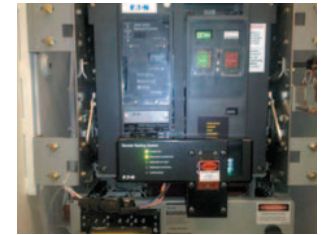
Remote Racking System
