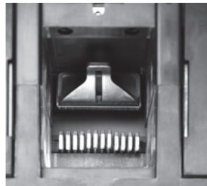
Magnum DS Breaker Contacts (Arc Chutes Removed)
