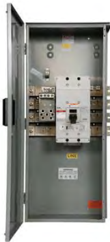
Main Circuit Breaker
