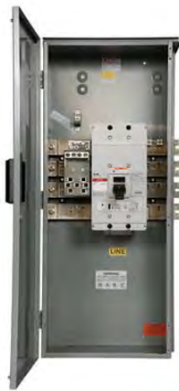
Main Circuit Breaker
