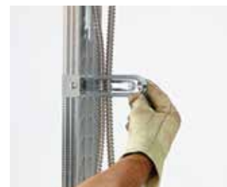
Once cables are inserted, wrap zip-tie around the end of the support to secure the cables
