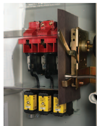
Enhanced Line Shield and Interlock Defeater
