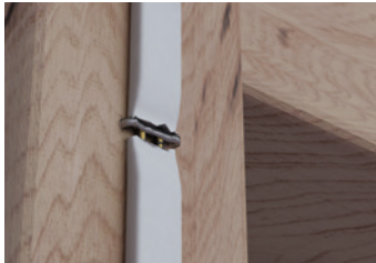
Tight staple can pierce insulation
